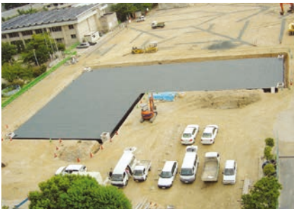
Fukuoka: Elementary school rainwater reservoir (storage capacity: 800m 3 )
