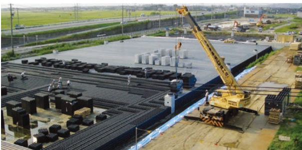
Ishikawa: Rezoned land rainwater reservoir (storage capacity: 9,200m 3 )
