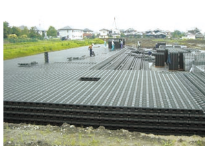
Aichi: Shopping center rainwater reservoir (storage capacity: 6,600m 3 )
